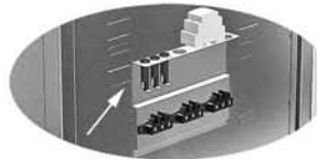
16/32A Commando Plug Fuses Location
